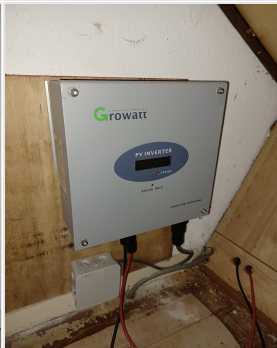
Inverter Growatt 1000S (na 1993)
